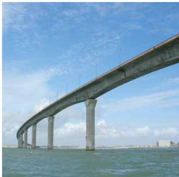
Some of the methods provided in the resource have been used to inspect and monitor prestressed cables on Pont Île de Ré. © Remi Jouan / Wikimedia Commons.
